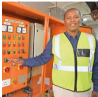
Let's switch it up: Mayoral Committee member for Water and Sanitation Cllr Siseko Mbandezi at a newly replaced electronic-control pump station panel.
